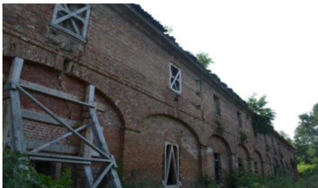
Figure 4 e 5 Front east (left) and North (right) of the building Riding stable Source: campaign photographic survey of Authors (September-October 2013)
